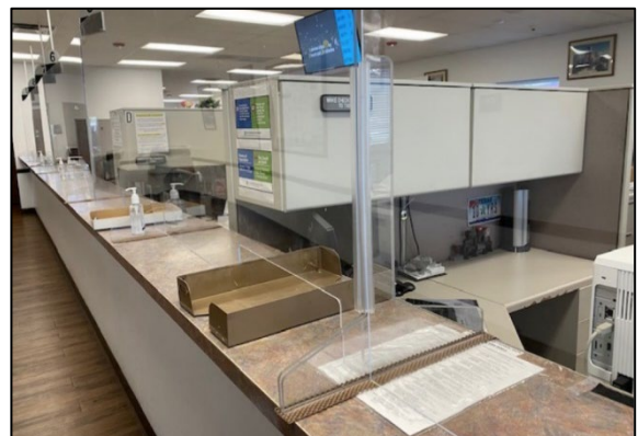
Plexiglass installed at the El Paso Regional Service Center.
